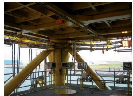
Fig 3. Actual positioning of GDU01 on offshore module
